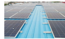
Solar Plant in Tin Shed
