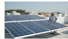
Solar Plant in Roof
